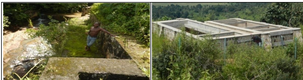
Figure 4. 10: Dilapidating water catchment(left) and purification tank (right)
